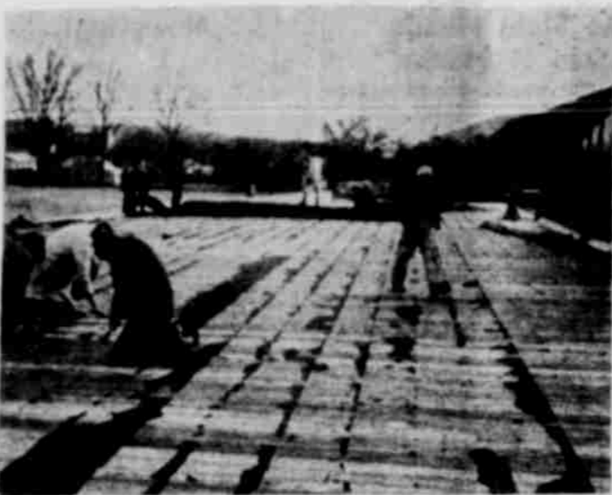
LIKE OLD MOTHER HUBBARD'S cupboard, the roof over the lone Cafeteria is "bare". Students clean up the tar paper and pull the nails preparing for the new roof. Identifiable is Mike Matthews.
