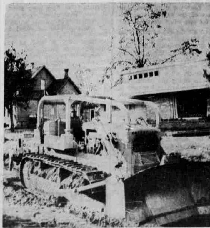
of the creek bed is lowered to the specifications that will carry the flood waters the size of the 1969 flood.
