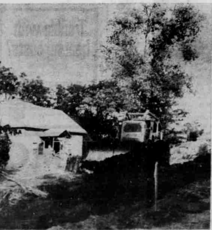
UP OVER THE TOP comes this cat to pile the dirt for mass shoveling into the dump truck. The other cat waits a turn to push dirt from the other direction. In this fashion the bottom
