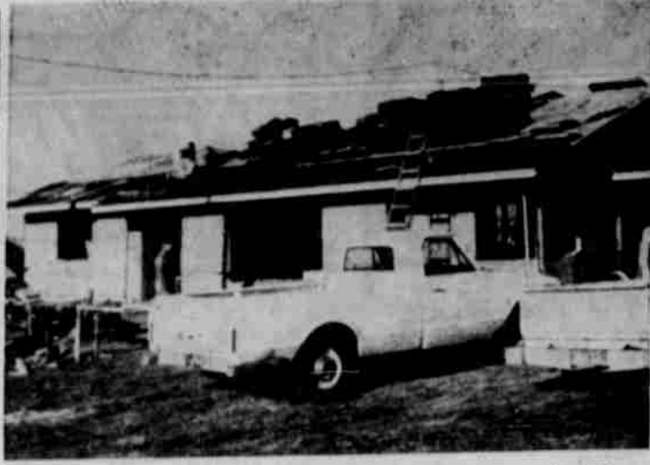
MAURICE GROVES and Howard Cleveland work on the Cleveland's house in sunny but below freezing weather.
