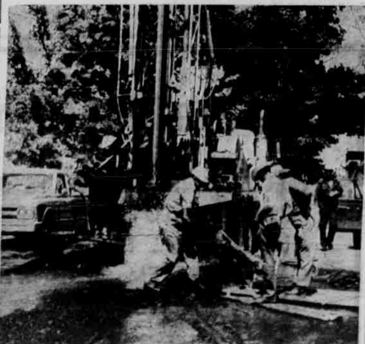
WATER, WATER EVERYWHERE . . . and it's all to drink and irrigate with. Fair board members are jubilant with the estimated 500 gallons a minute flow from the new well at the Fairgrounds. The well was completed shortly before the fair. The first activity is this Sunday with the all-day 4-H Horse Show beginning at 10 a.m.
