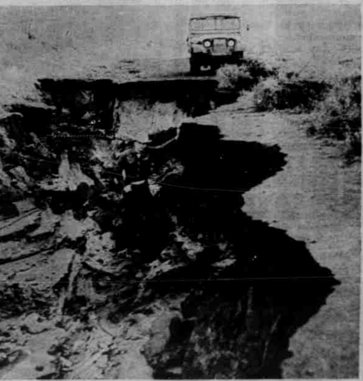
OOPS! Where's the road go? Major erosion on the county road between Al Bunch's and Judge Paul Jones' ranches left this gully, big enough to swallow Joe Wilhelm's jeep, last Sunday, Jan. 25. This is Kevin Dick's first photo and is the winner of five bucks for this week's Picture of the Week.
