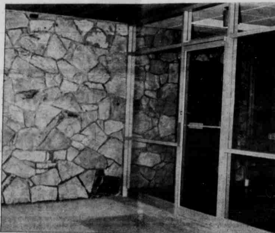
STONE FROM Eagle Creek Stone Quarries, Antelope, sets off entrance to the building and provides beautiful exterior finish.
