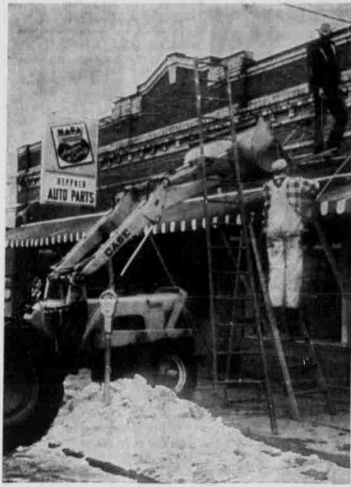
AFTER THE STORM COMES THE REPAIRS. Howard Keithley, standing on awning, and Bud Butterfield make repairs to the long awning in front of Wagon Wheel Cafe and Heppner Auto Parts. The awning dropped at the height of the recent storm under weight of heavy snow. It had been propped up temporarily since that time. (G-T Photo).
