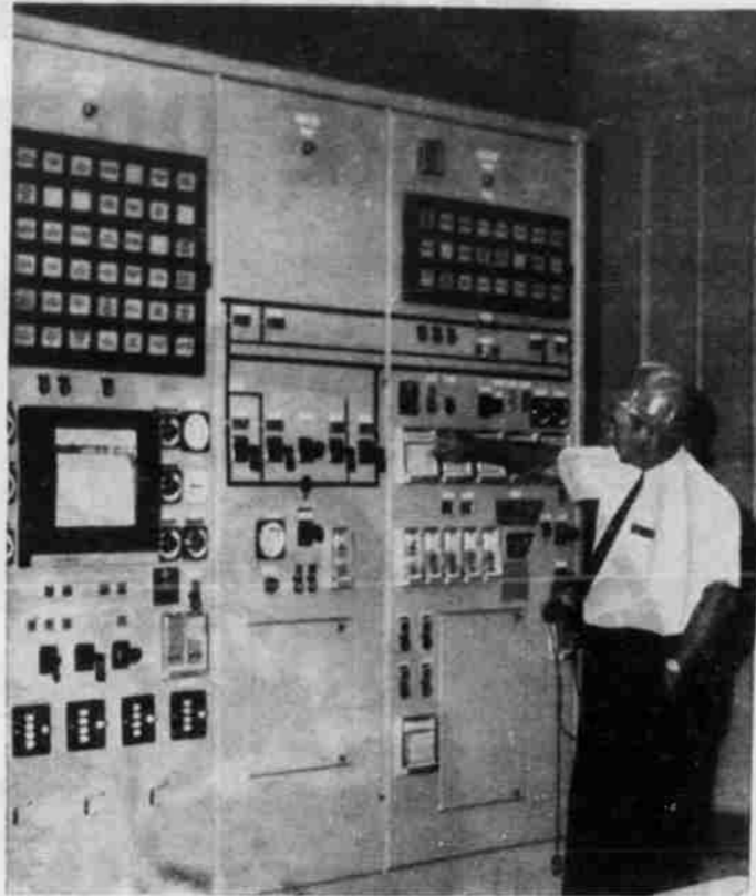
CHET BOND, Wallula, Pacific Gas Transmission Co. supervisor, explains the complicated switching panel at the PGT compressor station at Ione to members of the Ione Lions and the Heppner-Morrow county Chamber of Commerce at a tour of the station on September 23. Whenever anything goes wrong at the plant, a light comes on to indicate the trouble in one of the appropriate squares at top of the panel right and left. (G-T Photo).
