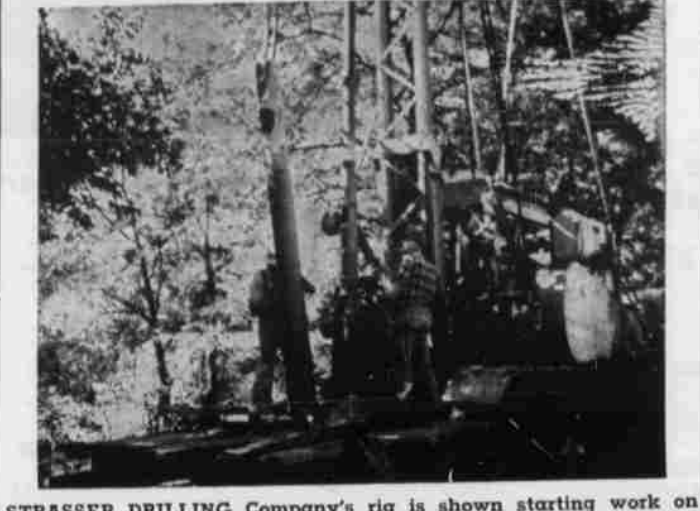
STRASSER DRILLING Company's rig is shown starting work on Well No. 1 at Irrigon, which has been in planning stages for several years. (G-T Photo)
