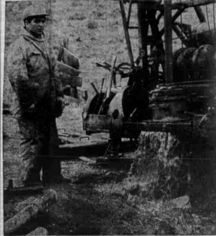
ENOUGH WATER to provide complete irrigation for the Willow Creek Country club is flowing from the new well brought in by Inter-Valley Drilling Co., Island City. The well is expected to produce 300 gallons per minute. Dan Ellsworth, who works with his father, Otto Ellsworth, in the company watches the flow. Dan attends Eastern Oregon College and is the 137 lb. conference wrestling champion. (Photo by Dr. Ed Schaffitz)
