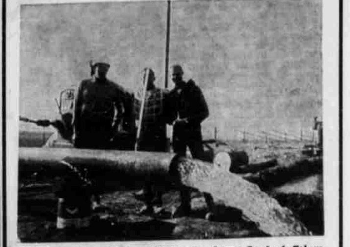
Bill Rice of Inter-Valley Drilling Co., Larry Byrd of Columbia Pump Co. and Ken Turner watch flow of new well at Turner Ranch.
