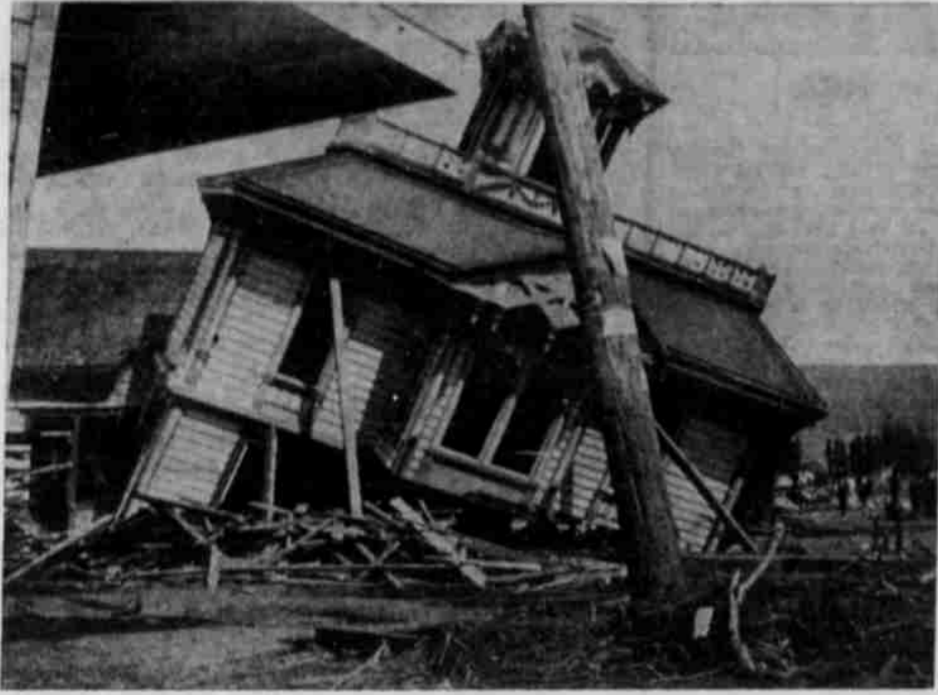
ON A SUNDAY AFTERNOON, when Heppner's devastating flood of 1903 struck on June 14, it did a pretty good job of wrecking the T. W. Ayers house which stood on Chase street a few lots south of the corner of May street. But the upper story of the house, minus the cupola and remodeled, was re-erected on Chase street to serve families for years to come. This is one of the most used of the well-known Heppner flood pictures.
