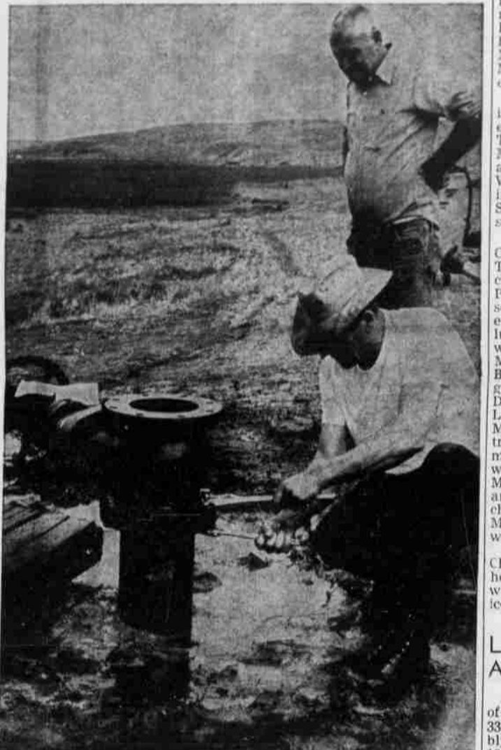
NO, THE ARTESIAN well didn't dry up on the Evans place. A drenched Don Evans in this photo has succeeded in capping the well and shutting off the flow. Roy French of Pendleton, who dug the well, stands by Evans. French said that he dug another well, also an artesian, with a smaller flow on the Dallas McDaniel place on Rhee Creek after digging the Evans well. When the Evans well produced a good supply at just over 230 feet, decision was almost made to stop there, but Evans decided to go deeper and the well came in as an artesian in just about 12 feet more. (G-T Photo).
