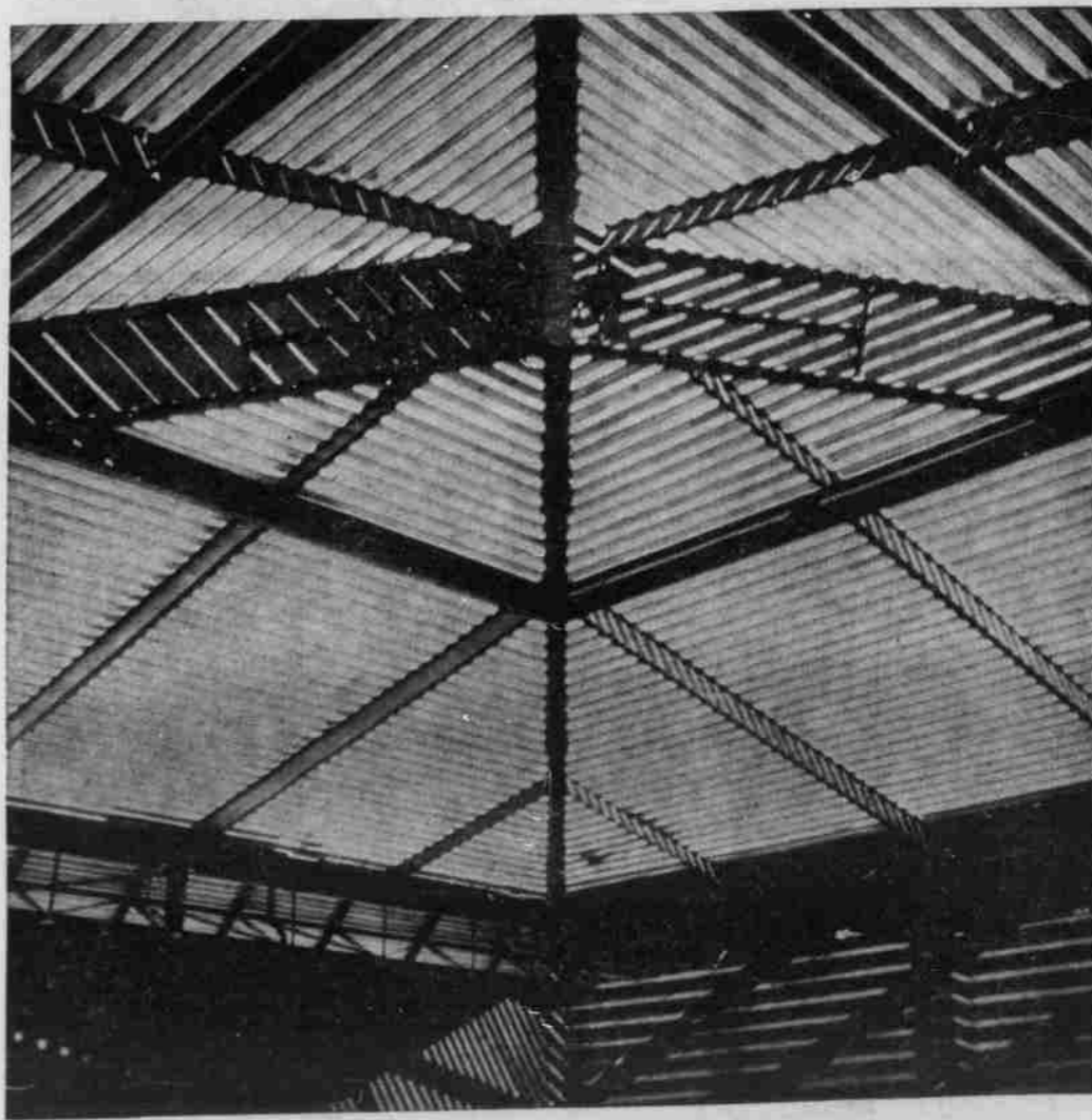
3. VIEW LOOKING to the roof from the gym floor brings out this group of geometric patterns. Shadows of the roof structure create other patterns on the gym wall at the bottom of the photo. Steps (not shown) lead down from student commons area to the gym, which is on a lower level than the rest of the building.
