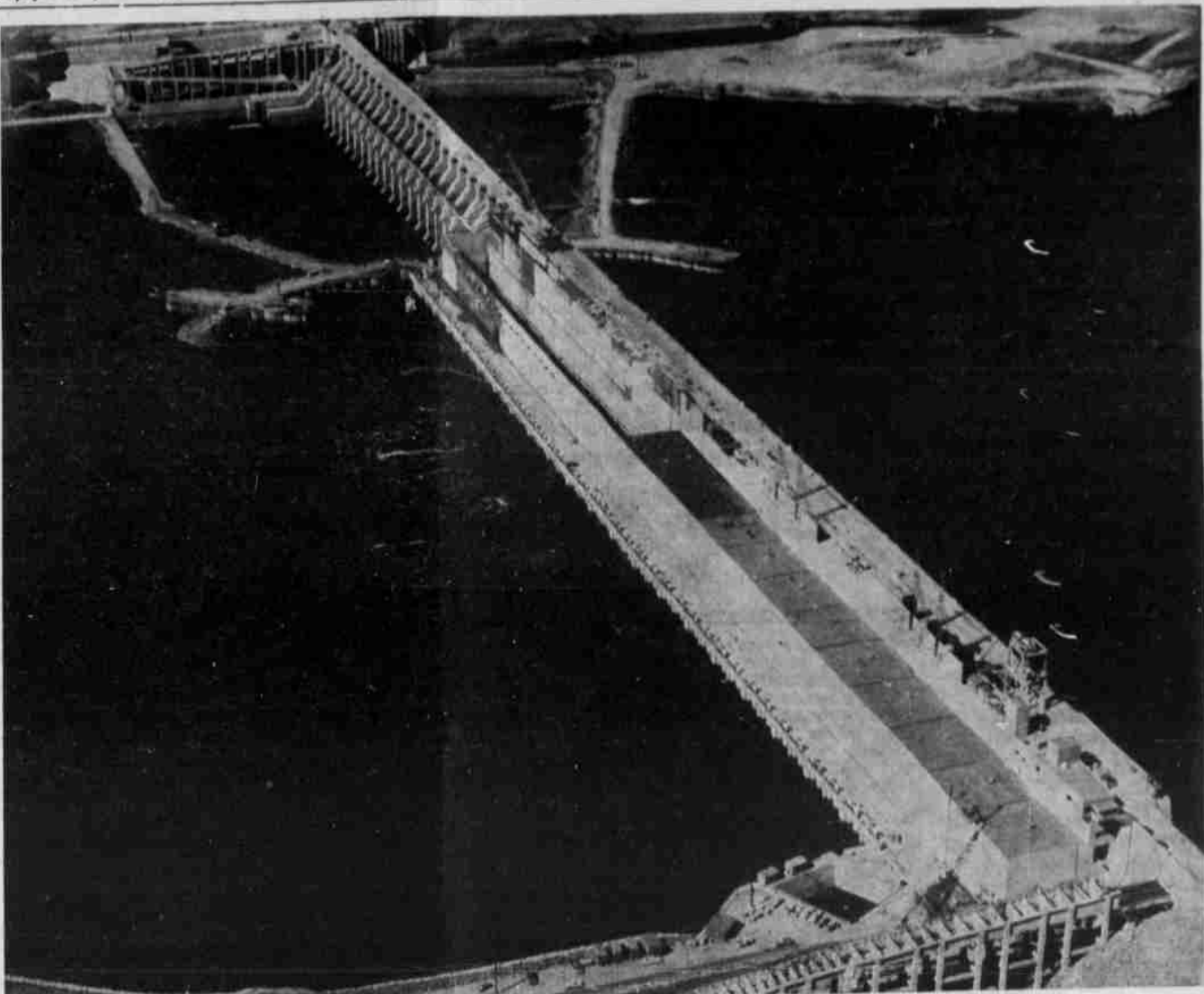
JOHN DAY LOCK AND DAM, under construction by the Walla Walla district, U. S. Army Corps of Engineers, near Rufus on the Columbia River, is shown with both cofferdams in place on the Washington shore (upper left). Pool level sills on the spillway will be raised behind the cofferdams, completing the dam which is scheduled to begin power generation in the spring of 1968. Oregon fish ladder is partially shown in the lower portion of the picture, with the 16-unit powerhouse extending to the spillway and cofferdams. The multi-purpose project will be the largest dam on the Columbia when completed. (Courtesy Hermiston Herald).
