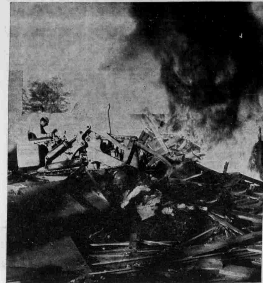
THE OLD BATH HOUSE at the Heppner swimming pool went up in flames last Thursday. After razing the building, the debris was burned against the concrete wall that was on the swim pool side. Many years ago, this was a power house that served Heppner. (G-T Photo).
