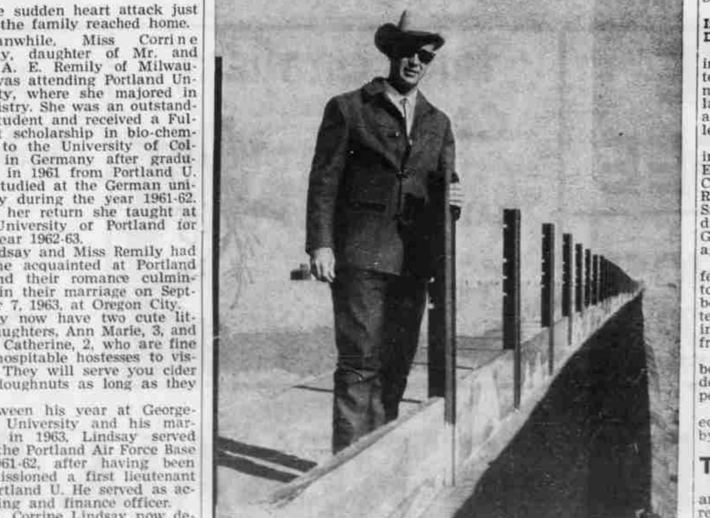
LARRY LINDSAY, Livestockman of the Year in Morrow county, stands beside a long feed bunk being completed at the home ranch. An 8 ft. concrete slab forms apron and foundation for the bunk. Pre-cast metal posts are sunk into the concrete. A total of 840 feet in this and another section are being added.
