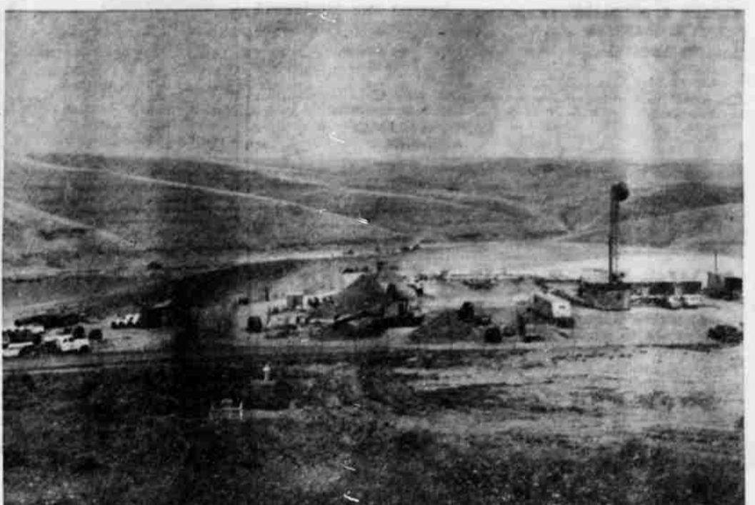
SITE OF THE new gas compressor station near Lone looks like "Construction Town, USA." with work moving right along on the $2,369,000 project of Pacific Gas Transmission. The station will increase capacity of PGT's pipeline to California. E. B. Schnell and Ray D. Kalal of Hermiston are contractors on the project.
