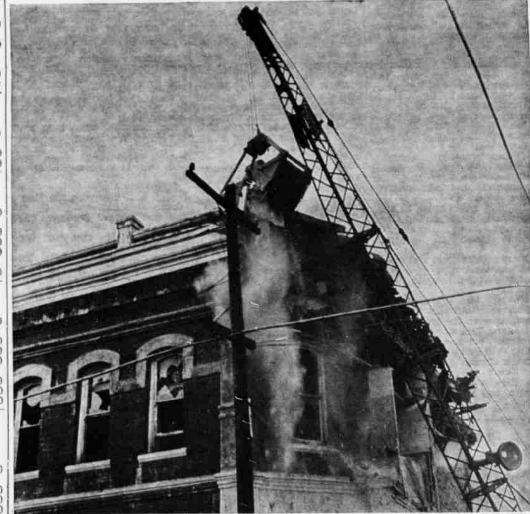
OUCH! Heavy steel bucket attached to the crane of the contractor demolishing the Case building scores telling blows on the soft sun-dried brick walls of the structure. Many came to gather bricks to use in yards and structures at their homes. (G-T Photo).
