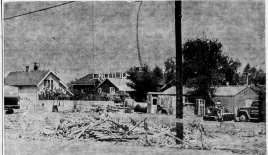
HERE'S ALL that was left of the once proud brick building at the corner of Main and Center streets when wreckers finished their demolition job. Process of leveling the site, preparatory to erecting a new service station, was underway recently. (G-T Photo).
