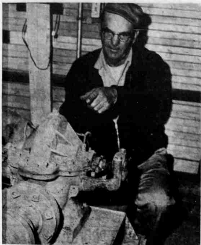
CITY SUPT. VIC GROSHENS points to the old pump at the swimming pool. This is part of the mechanical installations that would be replaced in rebuilding the pool. Voters will decide on the $110,000 venture at the bond election Wednesday, May 31. (G-T Photo)
