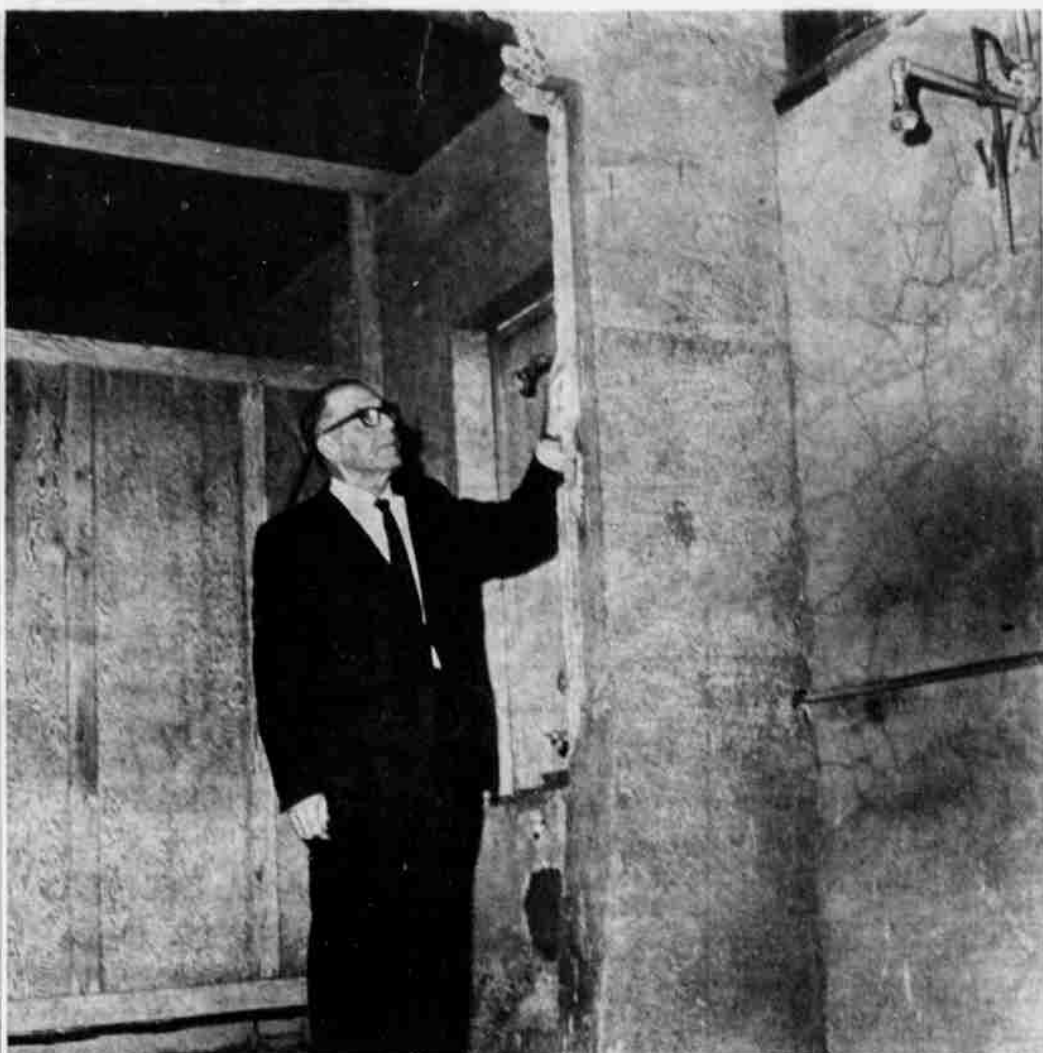
DINGY condition of the dressing rooms in the bath house at the Heppner municipal swimming pool is noted by Mayor Clarence Rosewall in this photo. Pool and bath house have been condemned by the State Board of Health. The building was converted to a bath house after serving as Heppner's first power house. Partitions (note in background) are thin and were designed so that they could be moved to use structure for recreation center at times when pool was not in use. (G-T Photo).
