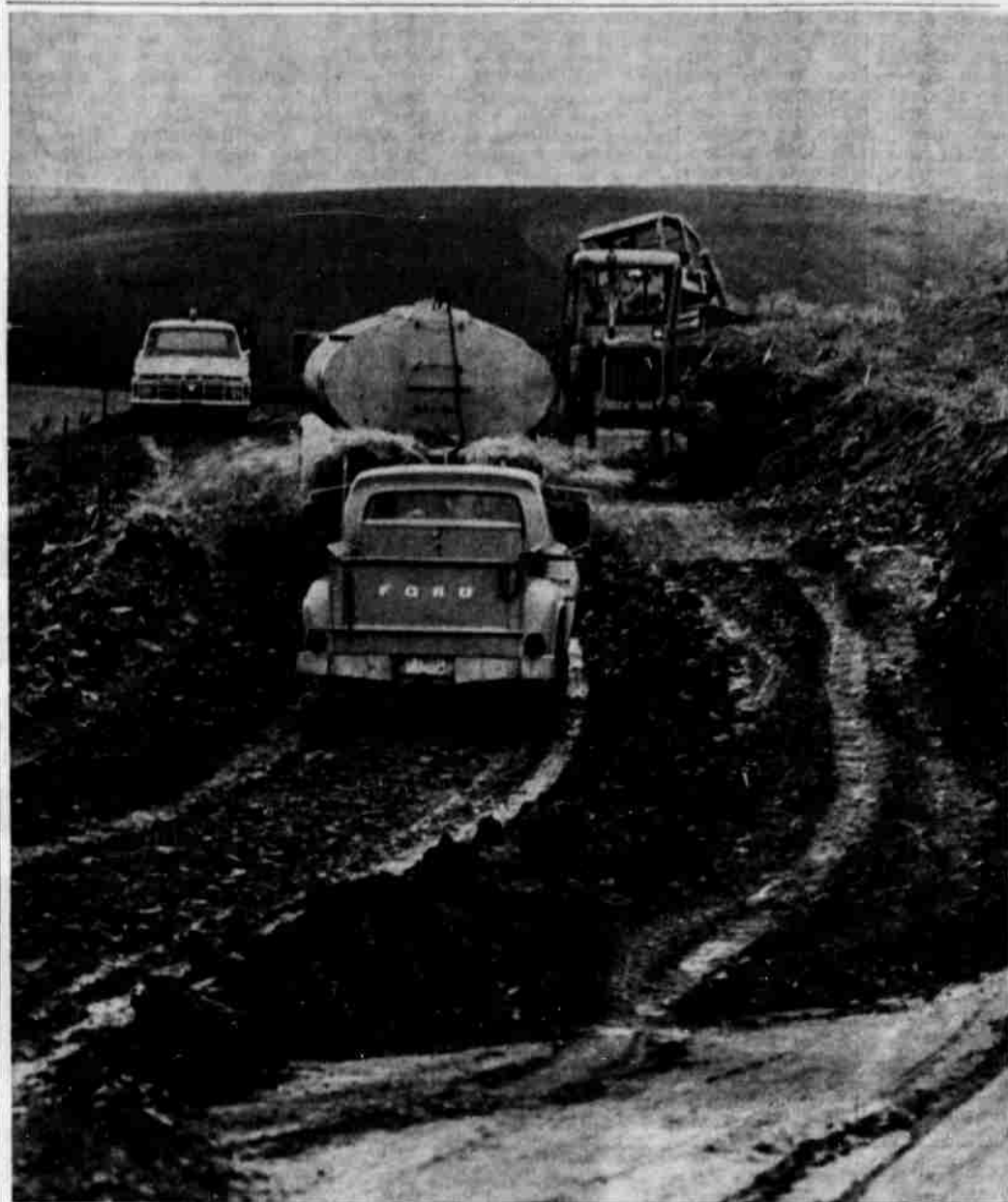
CONTRACTORS E. S. Schnell and Ray D. Kalal of Hermiston have had heavy equipment in operation to prepare an access road to the new compressor station of Pacific Gas Transmission Co. now under construction near Ione. The pickup nearest the camera is a PGT vehicle driven by Orville Reiber of the Wallula crew of the company. (Pacific Gas Transmission Co. Photo).
