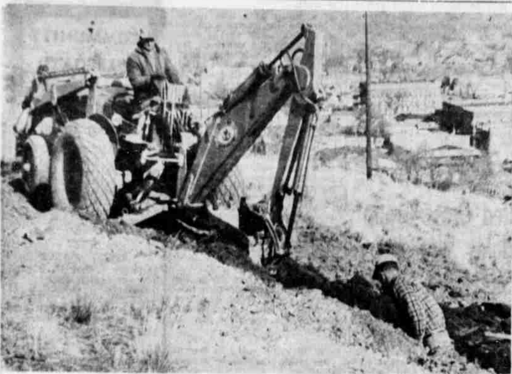
WORK IS NOW IN PROGRESS laying the water line around the hill on the west side of Heppner from the reservoir towards the high school. Bob Dobbs is shown operating the backhoe on the hillside while Wayne Harsin is at work in the ditch. The new line will give better fire protection to the school and offer better water service to the northwest part of town. (G-T Photo).
