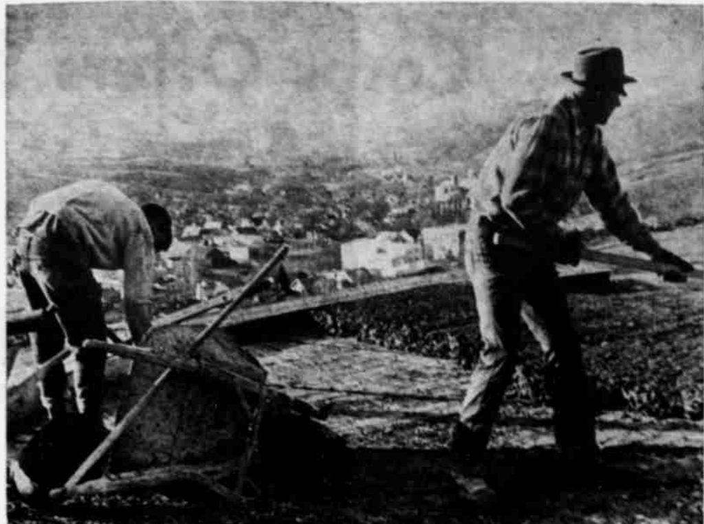
CONTRACTOR HOWARD KEITHLEY (Right) and his crew have a good view of Heppner (background) as they work at the county reservoir on the hill high above the courthouse. They are engaged in putting on a new cover and building up a wall of the concrete reservoir. (G-T Photo).
