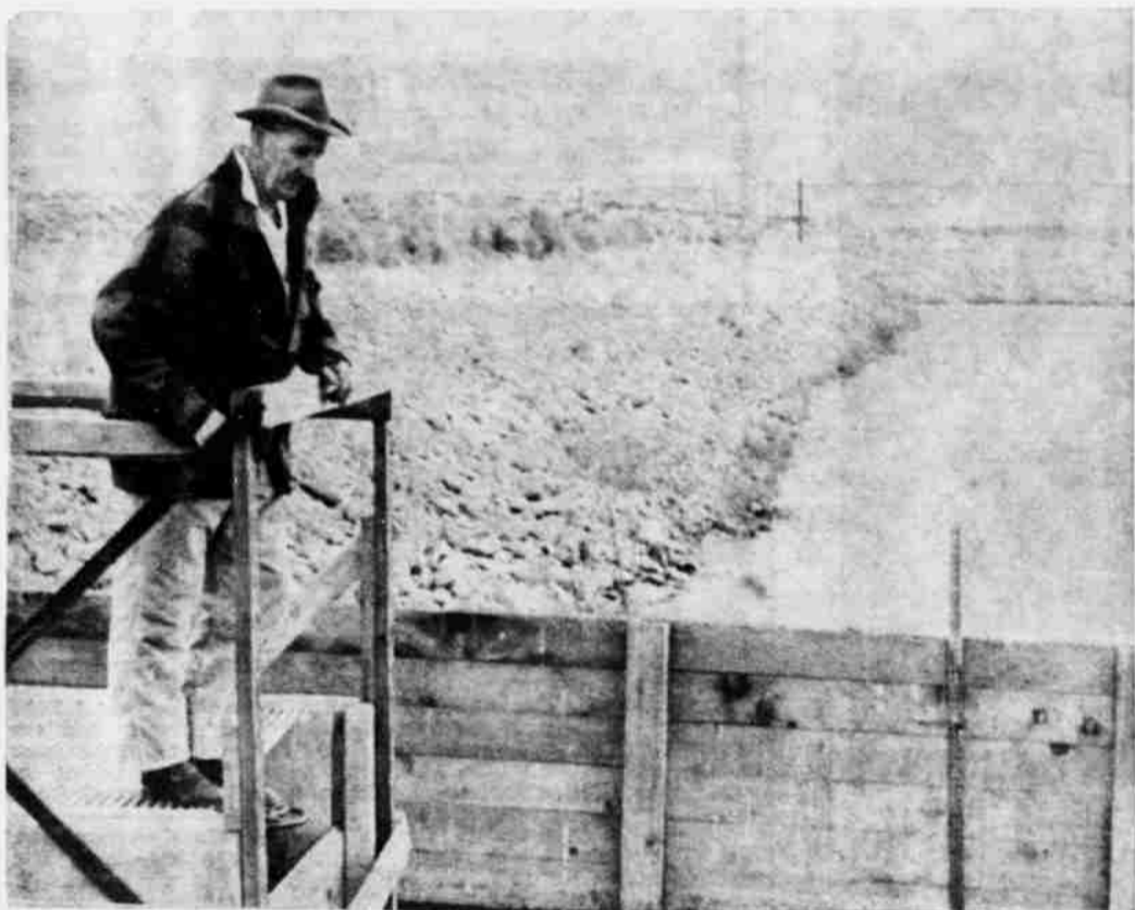
ZEARL GILLESPIE, public works superintendent at Boardman, checks operation of the sewer system at the lagoon handling effluent. The new Morrow county city has both a sanitary and storm sewer system.
