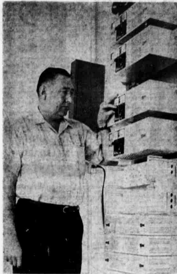
MICROWAVE RECEIVERS, just installed in the Heppner TV receiving station on the hill west of town, represent a considerable investment by Oregon Telecommunications, Inc., which will bring microwave TV here under contract, says Carl Spaulding, Heppner TV manager, shown examining the equipment. Barring unforeseen difficulties, microwave television may be in operation here in about two weeks. (G-T Photo by Spike Pardee)
