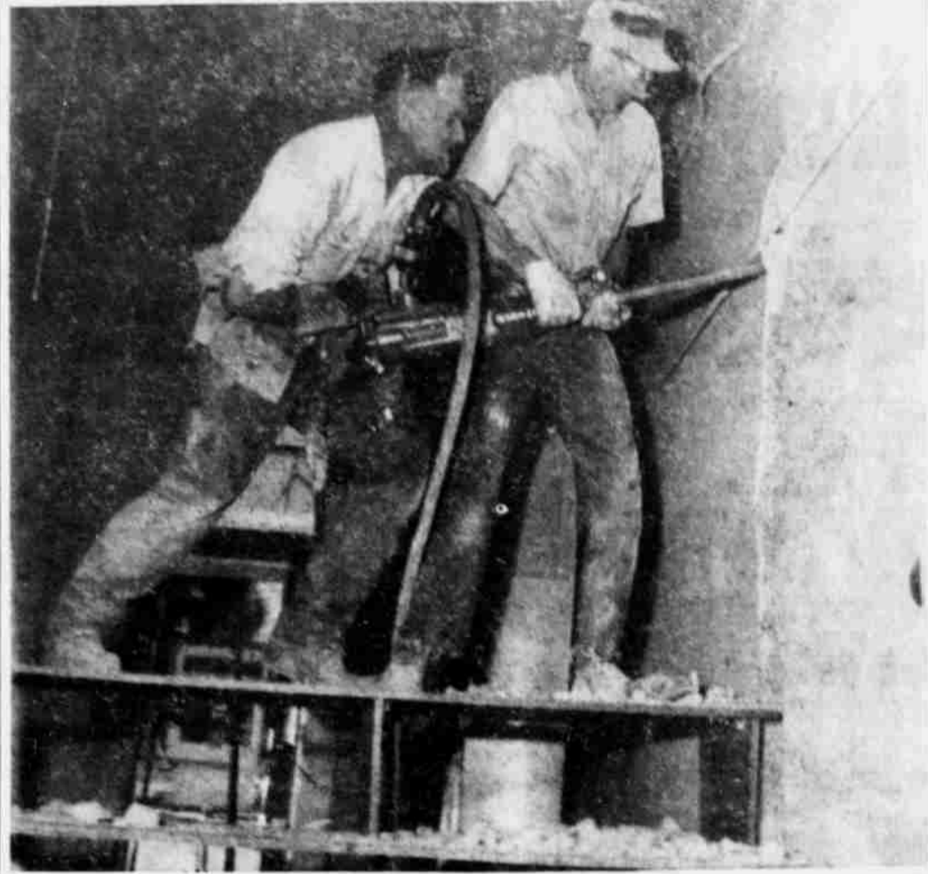
THICK CONCRETE WALL between the Gazette-Times shop and the Lanham building appeared to be as strong as a bank vault when Doyle Key, left, and Bruce Bothwell attacked it with a jackhammer Saturday. The picture doesn't show the beating the men took from operating the heavy hammer in a horizontal position, nor the dust that it kicked up. Noise from its operation could be heard pretty much throughout the business district. The Lanham building, occupied by the late Jos. J. Nys, attorney, for years, has been purchased by Mr. and Mrs. Wes Sherman and is now being converted into a new office for the newspaper. (G-T Photo)
