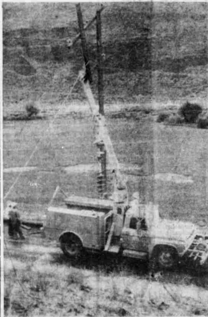
CREW of Columbia Basin Electric uses a new line truck with rotating boom on its first major job in the Rock Creek area above Olex Friday. One pole of the double structure was totally burned except for the stub left hanging at the cross arms. A conductor wire came out of an insulator and, in combination with the day's rain, caused a short and started the fire. Total cost of the new truck was about $18,000. Through using it, these major repairs were made without service interruption. A basket can be attached to the end of the boom to hoist workers to the top of poles. In the crew were Art Vance, Doyle Key, Bud Marshall, all of Heppner; Vern Wilson and Joe Poche, both of Condon.
