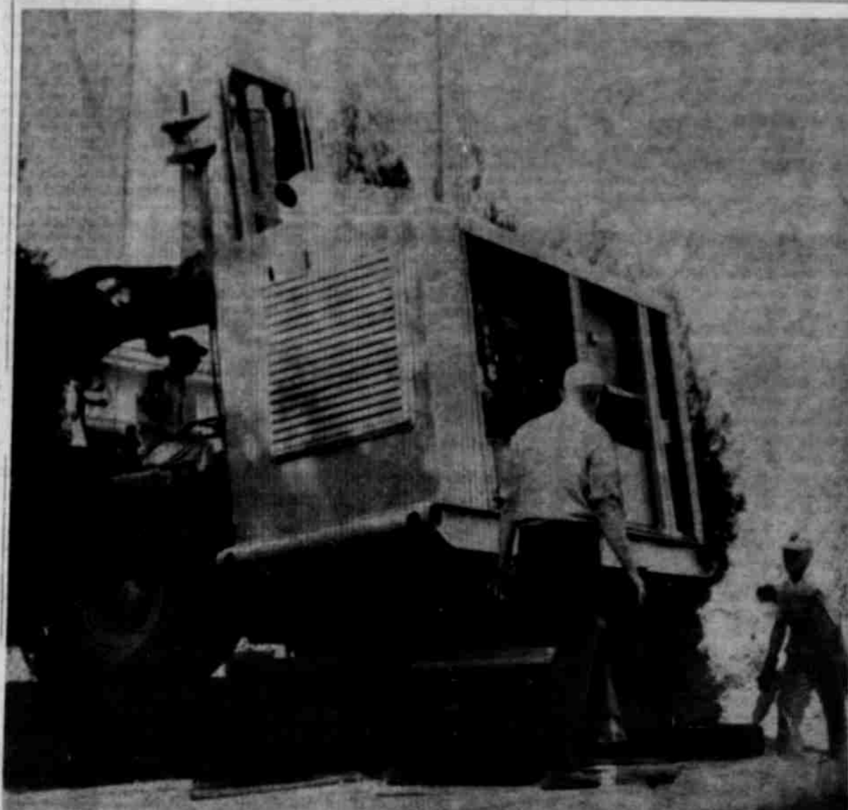
THIS BIG GENERATOR, weighing more than four tons, is being moved into place at Pioneer Memorial Hospital for use at times of emergency for power supply. Ned Sweek is driver of the fork lift truck. Elmer Moe is in the center, and Bob Lowe helps direct the job at the right. (Will O'Harra Photo)
