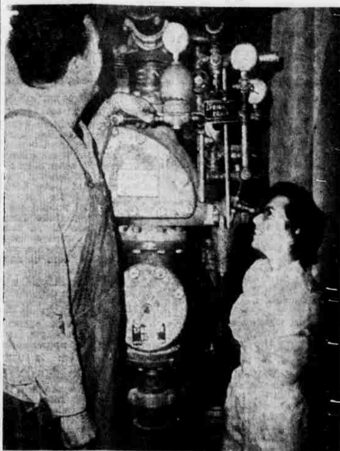
BIG GEORGE WHITEHALL, 6-4 and weighing "well over" 200 pounds explains to little Jane Mattair, nurse's aide at Pioneer Memorial hospital, some of the workings of the new automatic fire protection system at Pioneer Memorial hospital. They are standing by the accelerator valve which charges the line with water. The system throughout the original unit of the hospital was completed last week.
