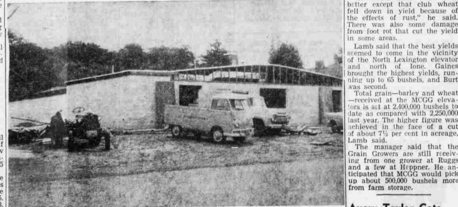
BOWLING ALLEY is taking shape in Heppner with building construction due to be completed soon by Wally Green, Hermiston, contractor. Installing lanes will be next step, and grand opening will probably be in early fall. (G-T Photo)
