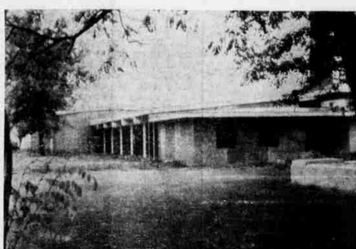
TREES FRAME the addition to the Houghton elementary school, Irrigon, now under construction. Existing building is to the right, out of the picture. In foreground of the picture is space for offices and auxiliary rooms, beyond which will be two classrooms and a library. The multipurpose room is visible at the left (rear) of picture.
