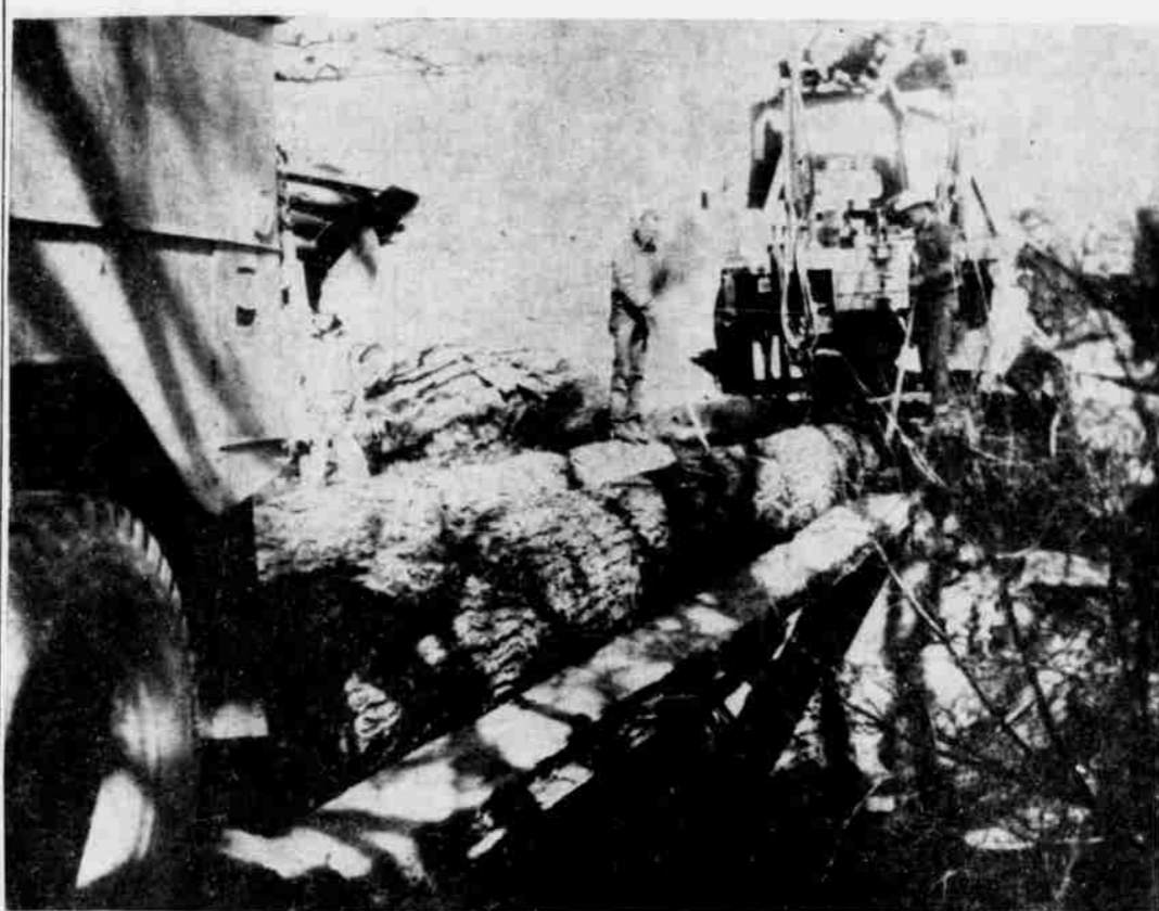
LOGS for the new bridge at Willow Creek golf course are shown being yarded into place last Wednesday by line trucks of Columbia Basin Electric Co-op. Truck at left hauled log into place by means of a cable while truck on the right slacked off on its cable. The trucks thus kept log suspended between them. Jack Loyd is visible standing on far end of the bridge. (G-T Photo)
