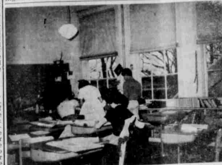
THIS PHOTO shows one of the classrooms now in use as an elementary room in the old Irrigon high school building, erected in 1921. The room is comfortably equipped, but has old-style high ceiling, old-fashioned windows and inadequate lighting by present-day standards. This room is on third level of the structure. Stairwell of the structure would act as a flue should fire break out in the building. (G-T Photo)
