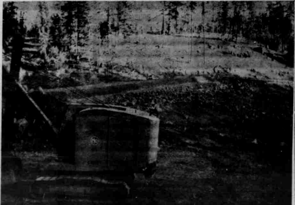
WORK OF constructing the earthfill dam at Bull Prairie reservoir, 45 miles south of Heppner, is near completion, as this photo shows. Layers of clay have been applied to the dam and road facing is now being applied. The reservoir will be one of the area's most popular outing and recreation spots when it is completed, filled and stocked with fish. Story on page 6 (G-T Photo)
