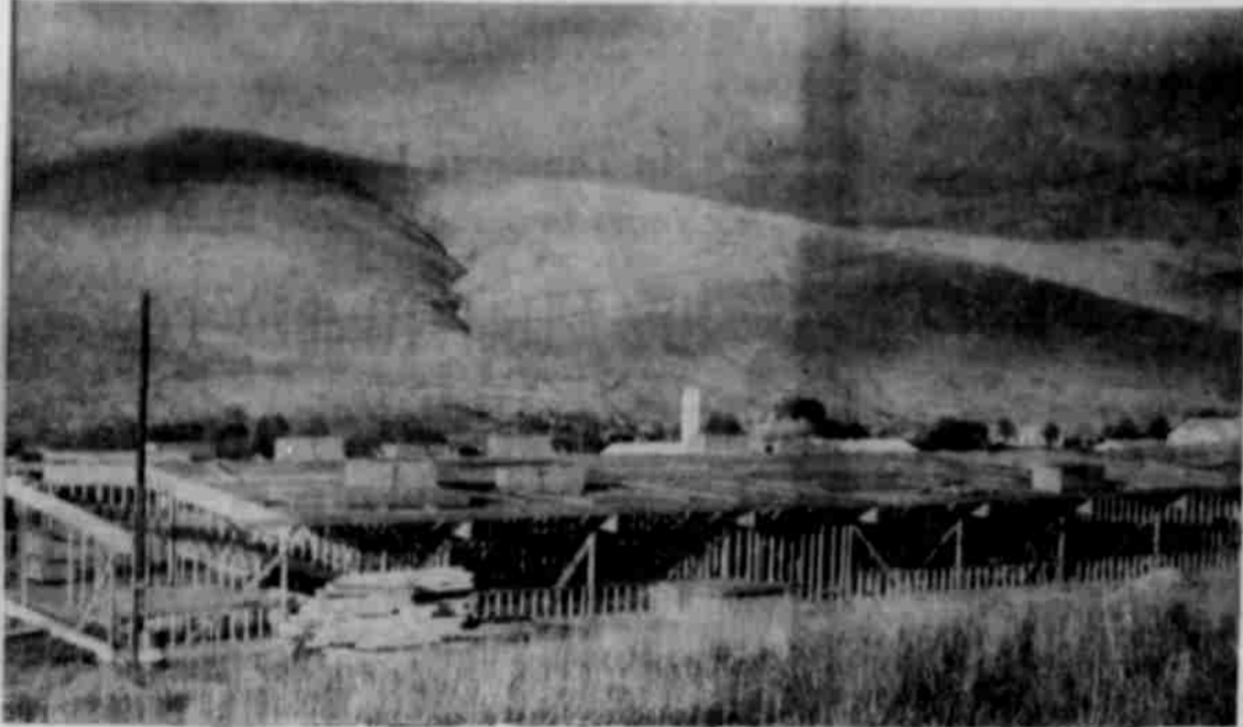
UNDER CONSTRUCTION on a site northwest of Heppner is this 8-room unit of a new school building. Designed for a high school building, it will be used at least for the first year as a grade school building. Before it may be used for high school purposes, science rooms, home economics room, library, multi-purpose room and additional classrooms need to be approved and constructed. The first unit is expected to be in use during the 1961-62 school year. (G-T Photo)
