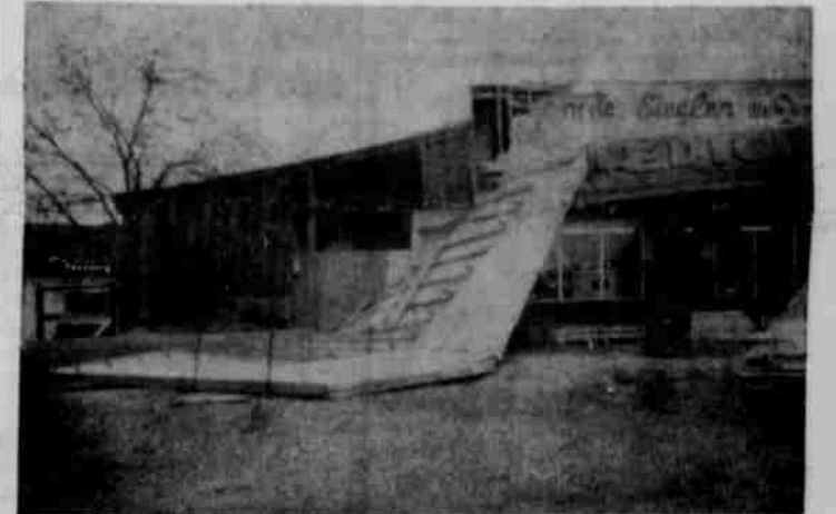
The E. L. Dick Appliance store as it looked last week following Sunday night's high wind storm. Damage was appraised at about $800. A new front on the warehouse section is almost completed.
