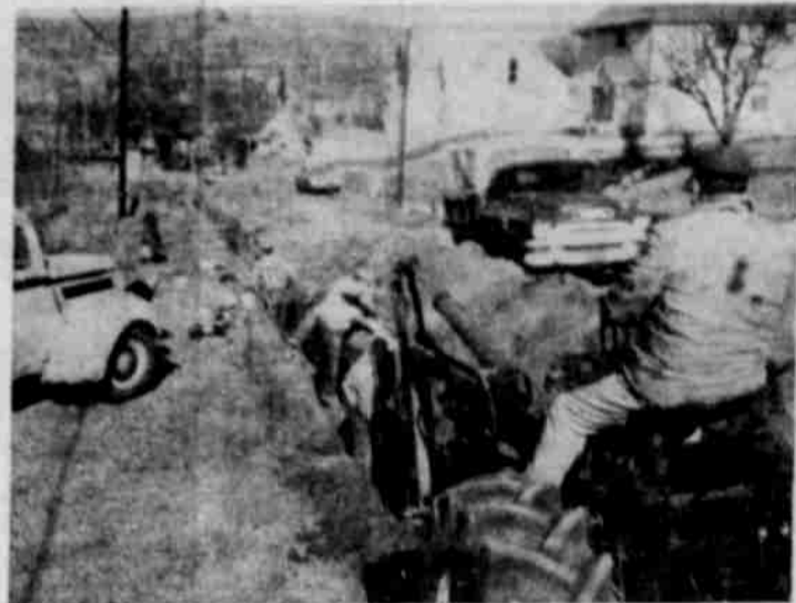
MORE WATER FOR RESIDENTS —City of Heppner crews last week started laying several thousand feet of new six inch water main which ultimately will give residents along the Condon highway and cemetery hill a greatly improved water supply. Here the pipe is being laid on South Main street and will extend to the south city limits. New fire hydrants on the line will also improve fire protection in the area. (GT Photo)
