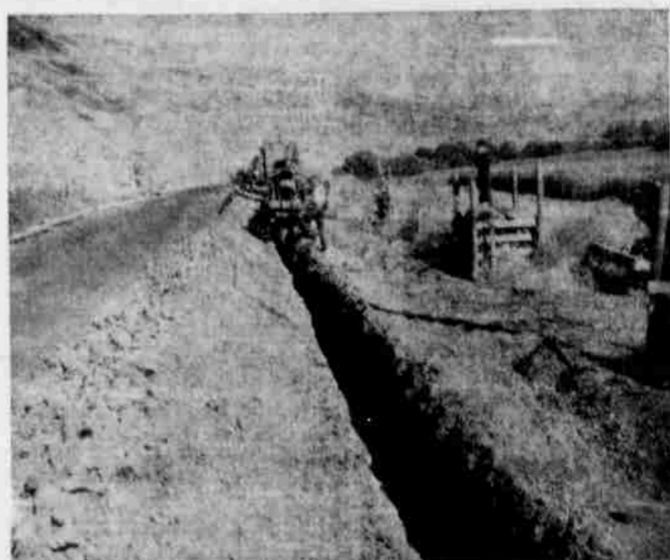
PIPELINE PROGRESSING—Crews of the Everett Den Herder Company are rapidly laying the six miles of the new City of Heppner water line along the shoulder of the Willow creek road. As much as 2000 feet of pipe has been laid in one day and Den Herder told the council Monday that if pipe is received on time the manufacturer, the job will be completed by early August. (GT Photo)
