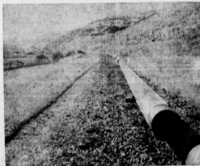
READY TO GO UNDERGROUND—A part of the nearly one-half mile of eight-inch steel pipe that is laid out along Willow creek ready to be placed in trench for new city water line. The laying of the six miles of pipe is now nearly 60 percent completed and when placed in use will help greatly to alleviate the city's water shortage. The new line will replace a like distance of old leaky concrete pipe. (GT Photo)
