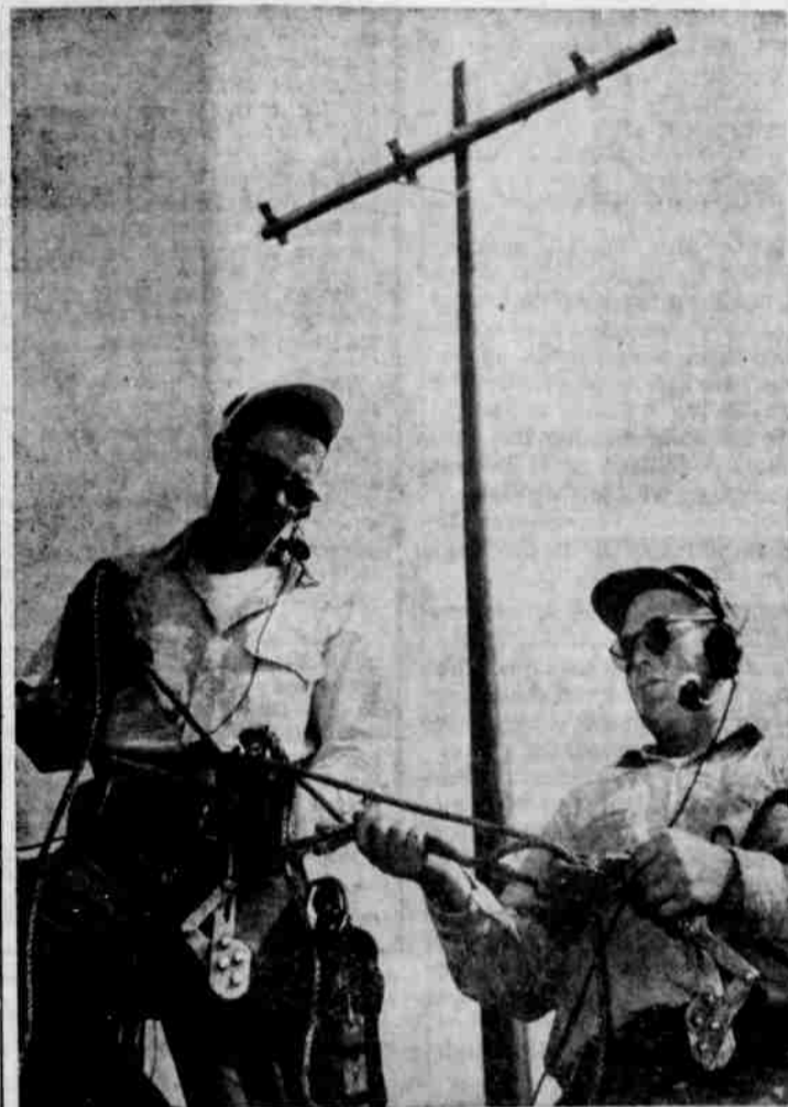
TELEPHONE LINEMEN, Bill Black, left, and C K "Chuck" Prinslow, pause to straighten their equipment which is used to put the proper tension on telephone wires being strung south of Heppner. Both men are from Salem. They are working on one of Pacific Telephone's largest rural projects in the state.
