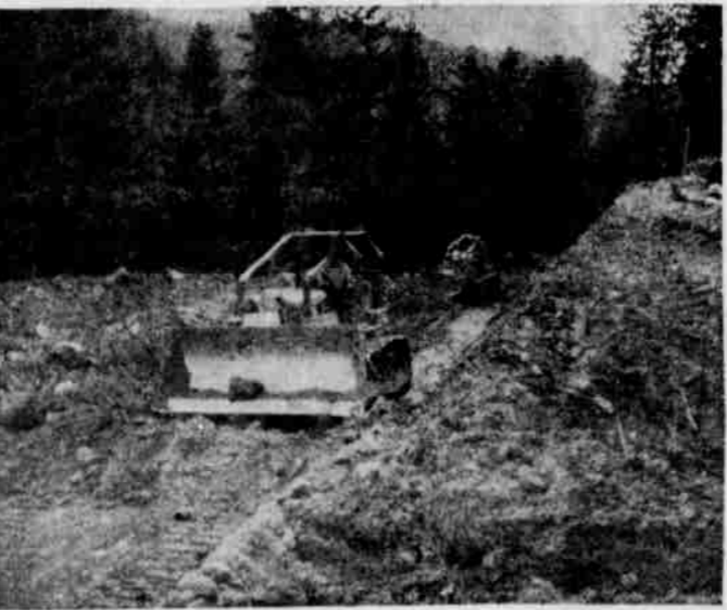
BIG DIG—Two of Heppner Pine's Cats are moving a mountain of dirt into a fill to take some of the many kinks out of the road. Considerable work remains to be done on the construction project, but trucking was started Monday over the route which is still a little rough in places for regular passenger cars. It is expected that it will be fall before the entire project is completed. The mill purchased about 16,000,000 feet of timber in this area which it is now logging. (GT Photos)
