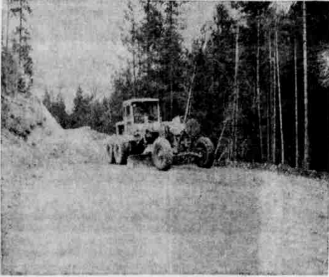
NEARLY 100 FEET WIDE in places, this section is five to six times the width of the old Shaw Creek road. The Heppner Pine woods crew has been rebuilding the road under terms of the Black Mountain sale of timber by the Forest Service. Here a grader is putting on some of the finishing touches.
