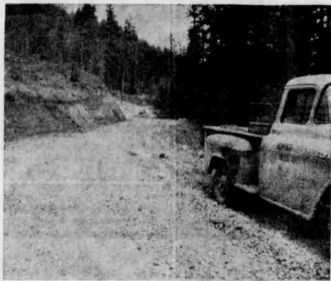
NEW ROAD UP SHAW CREEK GRADE, on upper Willow creek doesn't look much like the old one since Heppner Pine Mills crews started rebuilding the 3.7 miles of the narrow winding "cow trail" which used to carry the traffic into the mountains. This photo shows a section of the nearly completed road which will be rockd during the summer.
