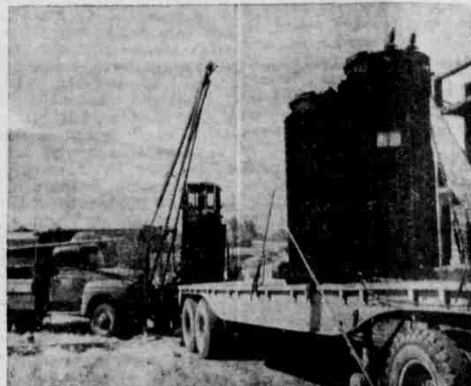
POWER OUTPUT DOUBLED —Workmen are unloading three big 500 KVA transformers at the Heppner substation of the Columbia Basin Electric Co-op which will double the capacity of the plant. Each of the transformers weighed about five tons and will work at 69,000 volts. This is the first of three substations on the REA system which is being enlarged to carry increased load. At the present time the average consumption of electricity on farms served by Columbia Basin is 1300 kilowatt hours per month, one of the highest in the state. (GT Photo)
