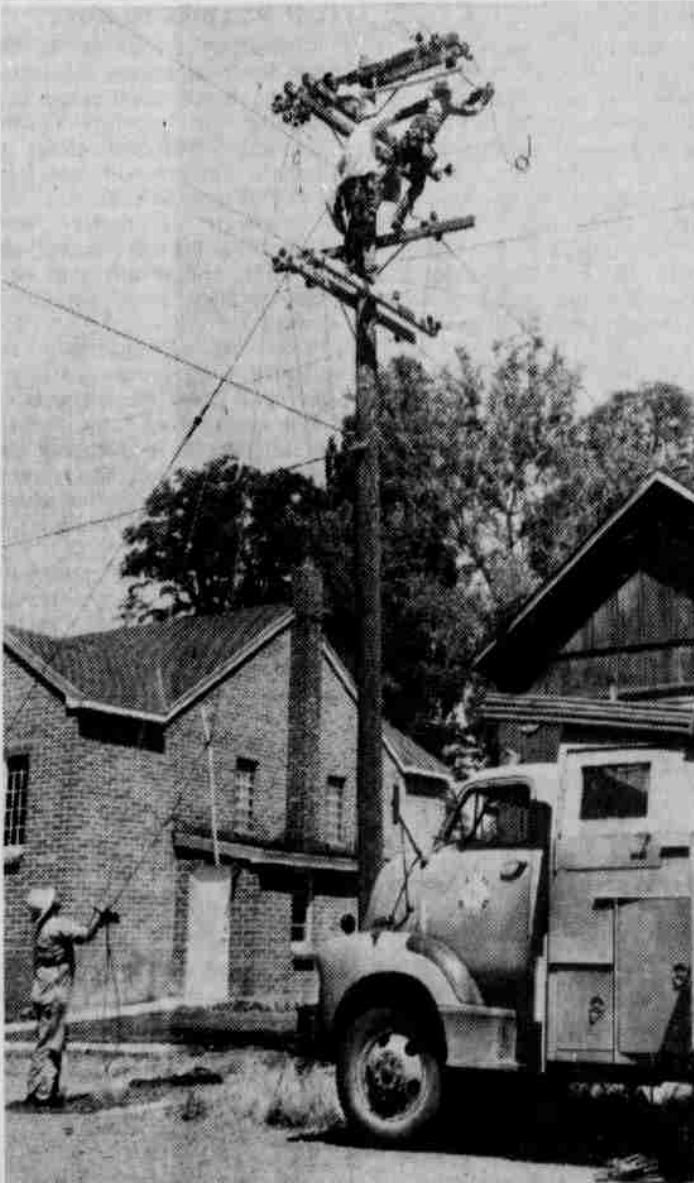
PACIFIC POWER and Light company is now working on a major power voltage improvement in the Ione area which will greatly improve and strengthen the area's electric service. Shown above, as they make ready to convert a section of residential line, are PP&L linemen Fred Sanders, top right, foreman, and Walter Bryant, while Scotty Walters assists from below. Voltages in the area are being increased from 2,400 to 12,000 volts.
