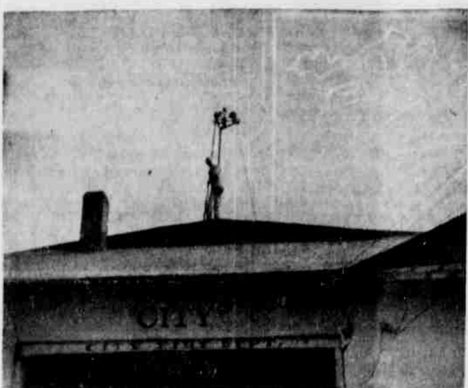
LITTLE BUT LOUD —Completing the job of installing the Heppner Fire Department's new air horn fire alarm is James Angell, shown here standing on the tower atop the city hall. The new horns are soon to be put into operation to call firemen and it is expected that they will be heard distinctly in all parts of Heppner. Department members had hoped to use the horns for the first time Tuesday during the Civilian Defense test alert, but mechanical troubles with new compressing equipment delayed their operation. When operating, they will be used in place of the present siren which has proved inadequate, and tests will probably take place within the next few days. The siren will be kept for flood warning or standby use.
