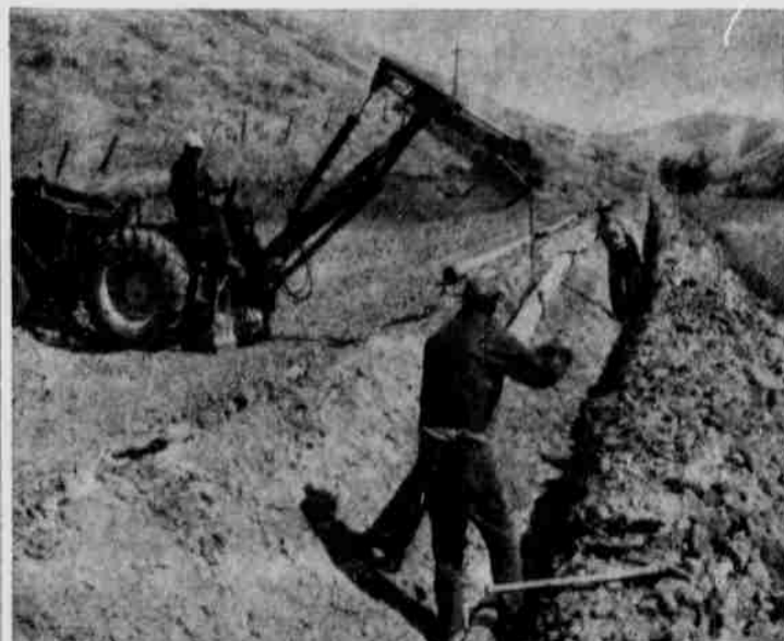
NEW WATER LINE goes into the ground as crews are nearing the completion of the project which renews two miles of Heppner's main water line from the Willow creek wells. Shown are Vic Groshens, city superintendent, foreground, and Frank Hamlin reading the section of 8 inch pipe for laying. Handling the digger is Bob Debbis. The crew hopes to complete the work by this weekend.
