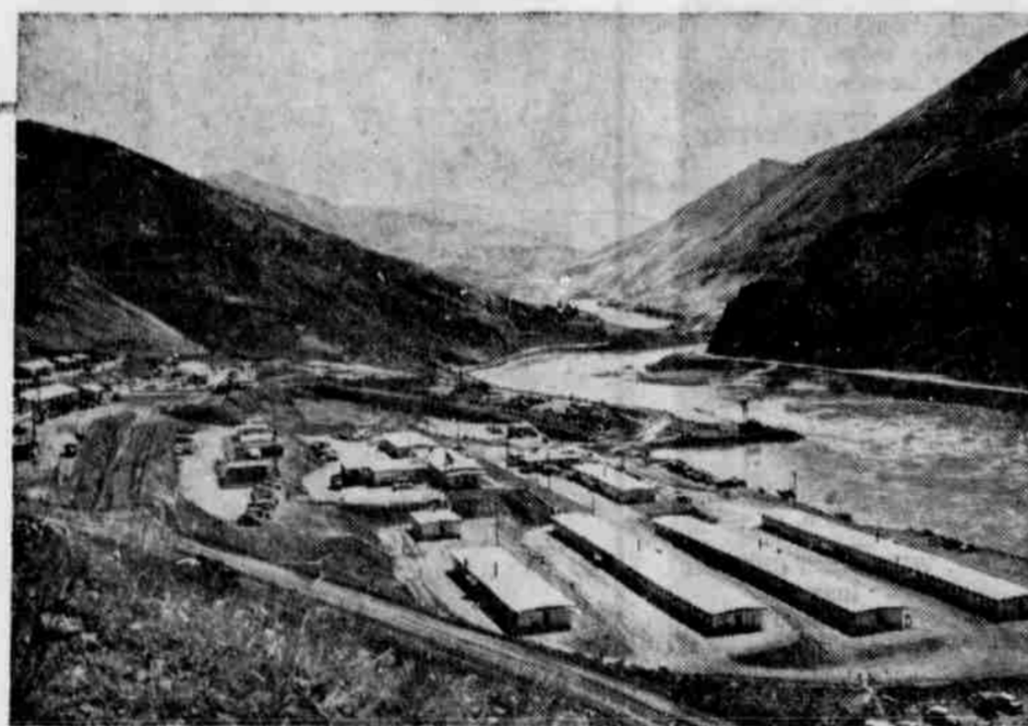
On the job at Brownlee dam site are 800 construction workers. River soon will be diverted through a tunnel and the dam will rise 395 feet above foundation level. Project will be completed late in 1958.
