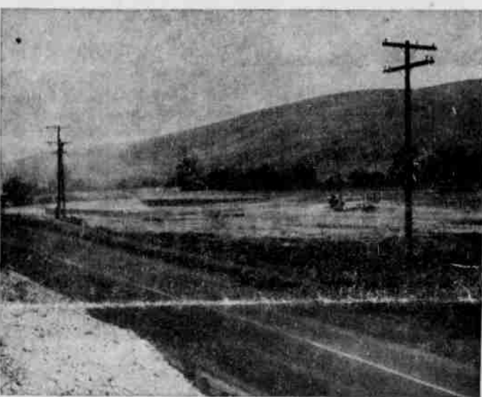
NEW SITE—This fall the United Stud mill will be moved to this site now being prepared just west of Heppner. In the center of the leveled tract can be seen the mill pond adjacent to which the mill will be built. The equipment to the right of the pond is part of the planer which will be housed in a steel building. (GT Photos)
