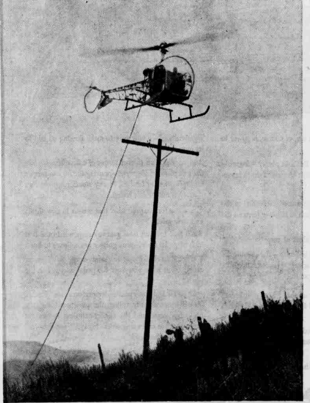
"Birlybird" helps string a telephone line. More and more uses are being found for helicopters in the telephone business. Not long ago, one was used to help a tele-crew string over two miles of wire across several steep canyons loaded with brush and poison oak. After poles were put up on the hill tops, the 'copter laid a rope across the cross-arms. Then the wire was fastened to the rope and the crew pulled it into position from pole to pole. In this way, a job that would have taken a week was done in an and a half. Corner-cutters like this do a lot, of course, to speed up the expansion of telephone system. The men and women of Pacific Telephone work to make telephone more useful every day.
