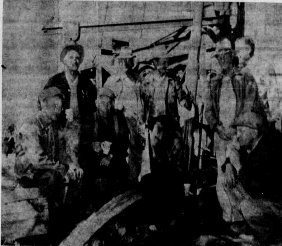
EVERYBODY'S HAPPY as they watch 700 gallons per minute of good cold water pour from the new Ione city well. Gathered around to watch the completion of the 24 hour test are left to right Eldon Tucker, Gus Janssen, driller; Noel Dobyns, Oscar Lundell, Roy Lindstrom, Harry Yarnell, Ed Bristow and mayor Omar Rietmann.
