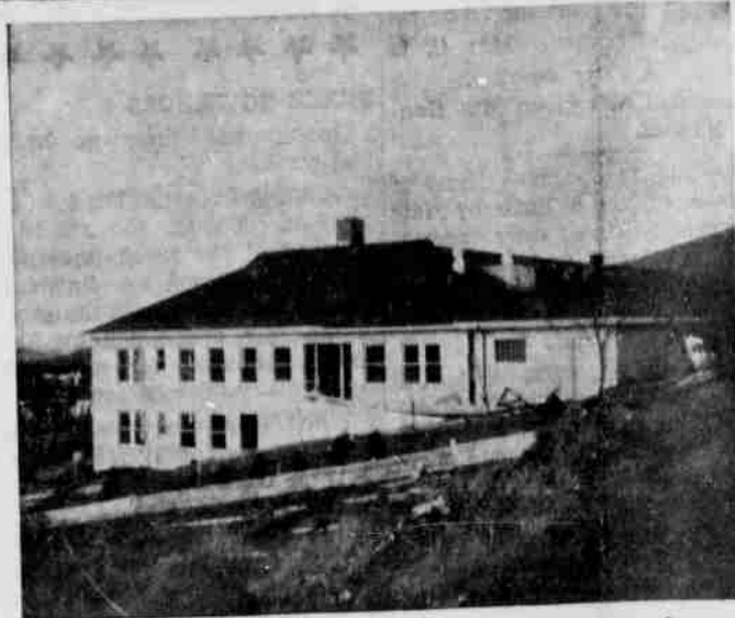
NEW HOSPITAL ADDITION is rapidly taking form as workmen are now putting the finish on the outside of the wing which adjoins the building on the south. The new unit will provide badly needed additional bedrooms and space for a health center and offices for the county health nurse on the lower floor.
